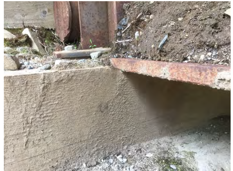
Left abutment timber sill 10mm crush
